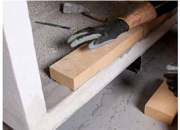
Bed the firebricks on to a 3mm layer of firebrick mortar. Use the tables on the previous page as a guide.
