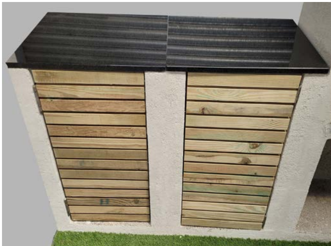
Place the second granite surface on the logstore and ensure these are level.
