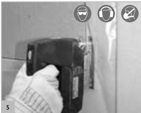
5 Make the opening. NOTE: Load Bearing elements must not be weakened! IMPORTANT: follow the safe working notes on p.35.
